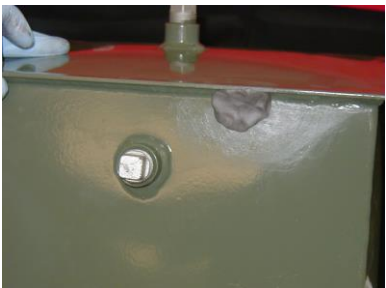
Apply Polywater ® Putty Stick ½ inch beyond leak; ⅛ to ¼ inch thick
